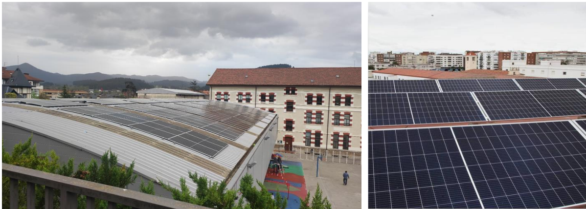
Figure 20 - Gernika's installation in the roof of the school (a). Photovoltaic panels (b)
