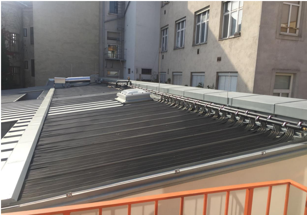
Figure 4 - Solar thermal mats in Vienna
